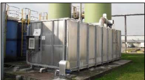
Figura 18: Biofiltro AirClean E2
