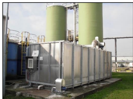
Figura 15: Biofiltro AirClean E2
